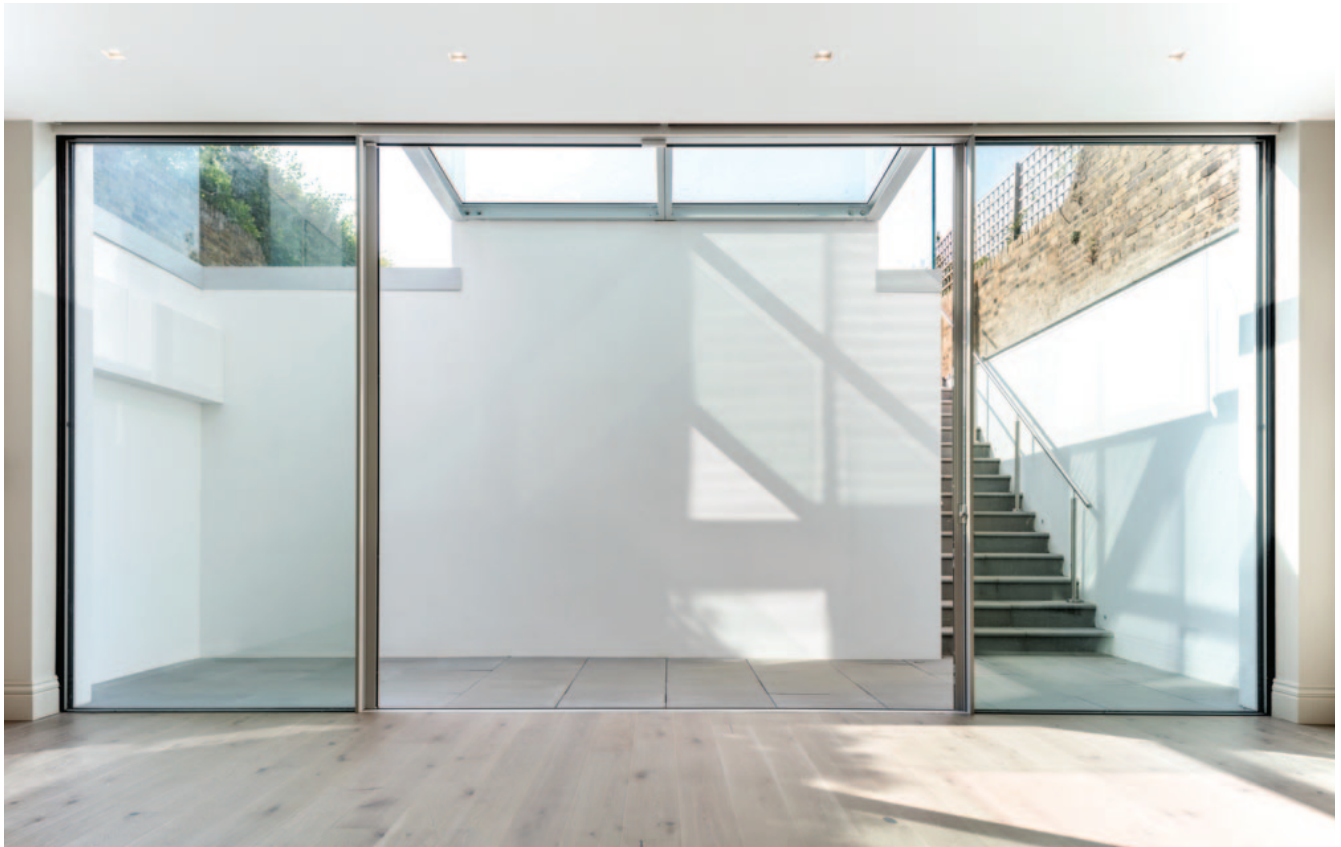
This is the basement view of the opposite Fusion Vista 19 installation. The walk-on glass roof light allows the light to flow into the basement area.
